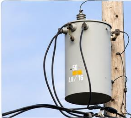
Image B Pole-Mounted Distribution Transformer
