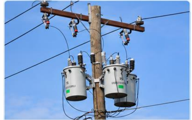
Image C Pole-Mounted Transformer Bank
