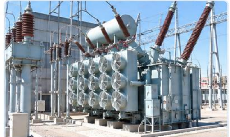
Image F Substation Power Transformer
